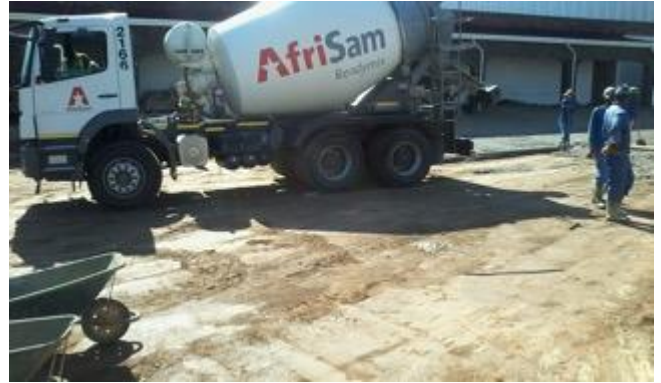
Uplifting of old paving and reinstating in a different area, concrete placement and site management
